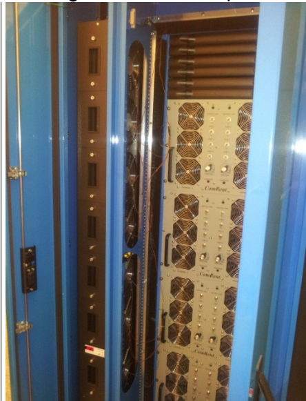
R.A.S.E.R. HD additional sensors, load-banks and one exchanger
